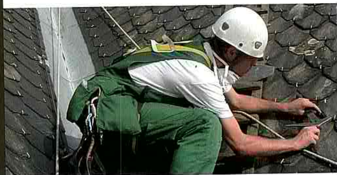
Regular maintenance with minimal intervention: Monumentenwachter replacing broken tiles on a roof.
